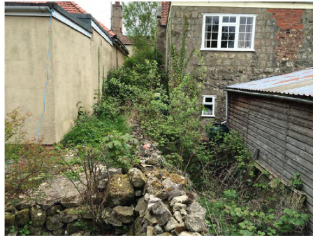
View to show the retaining wall on the site boundary to Merton House
